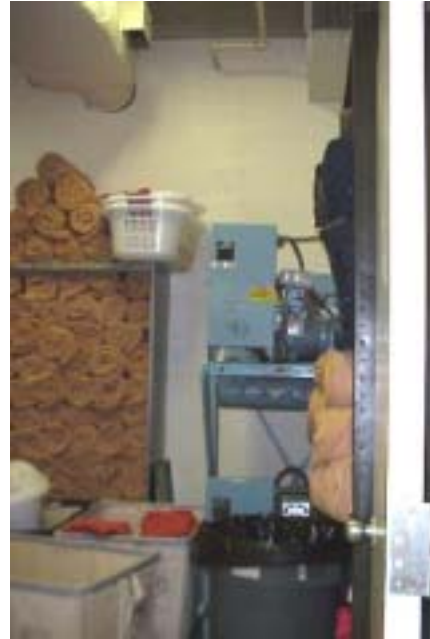
Figure 11 Mechanical Equipment in Laundry
