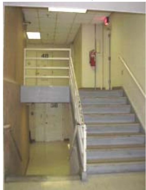
Figure 11 Impact of Unequal Floor Elevations (Old Jail to Expansion)
